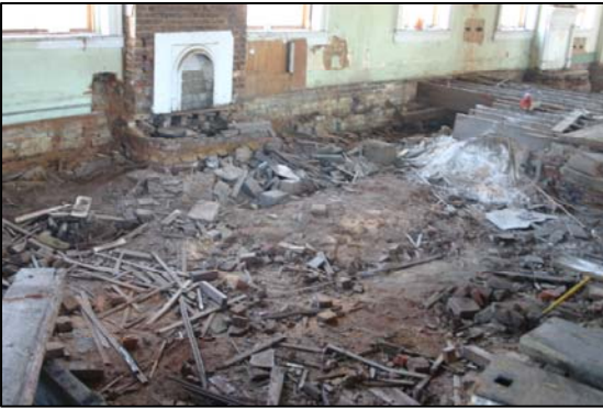
Fireplaces were collapsing, and walls in danger of falling when work began on the 1869 courthouse
