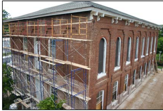
Thousands of bricks were repointed during the project, and balconies returned to the front and rear of the building
